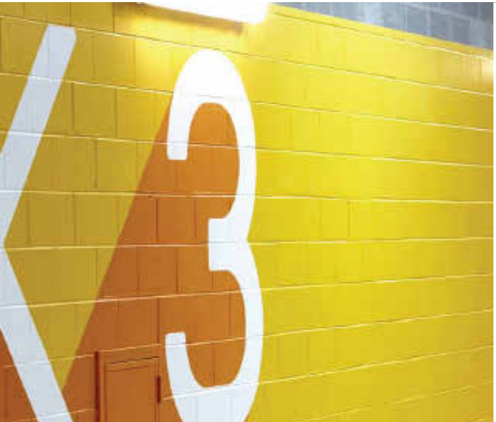
WA PT FACADE DETAIL: INDICATIVE ORANGE PAINT
